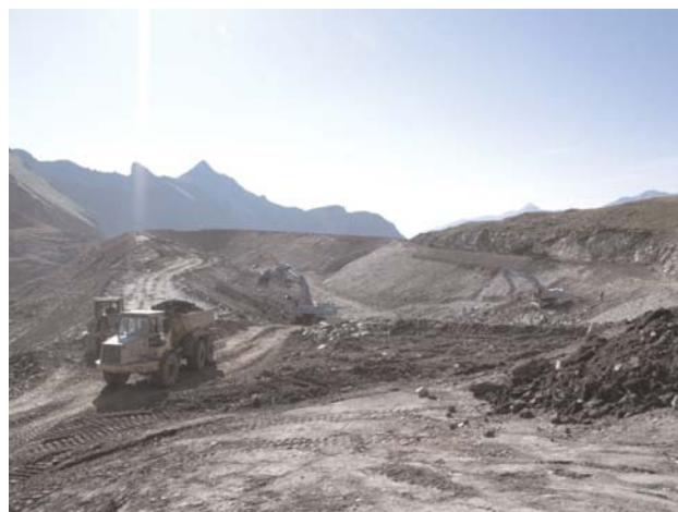
Figure 1: In the second year of the trial (2005), interventions continued at the trial site, for example a storage pond was built in direct vicinity to the trial site
