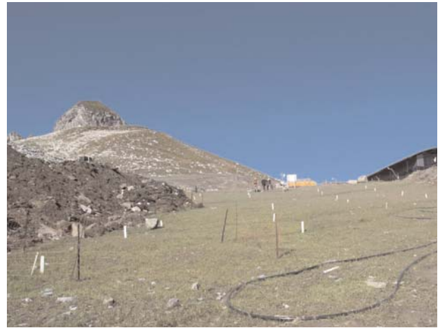
Figure 2: The trial site Obertauern in September 2005: The influence from ongoing construction work is obvious. On the left side, it is the construction work of the storage pond (see Figure 1 )
