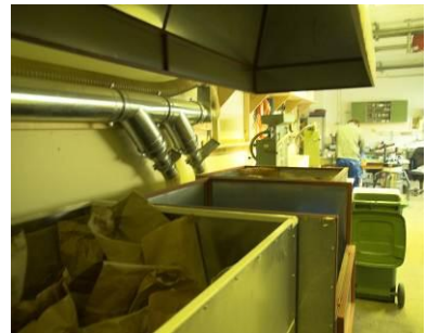
Figure 27: The drying system with hot/cold air at AREC
